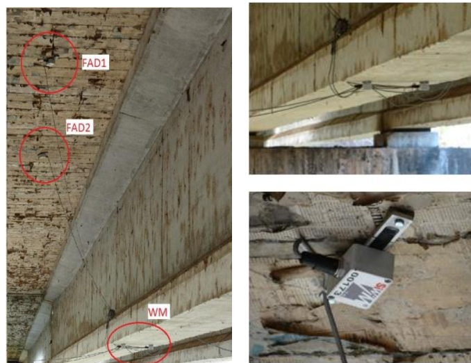
Figure 2 – Instrumentation position of the B-WIM sensors
